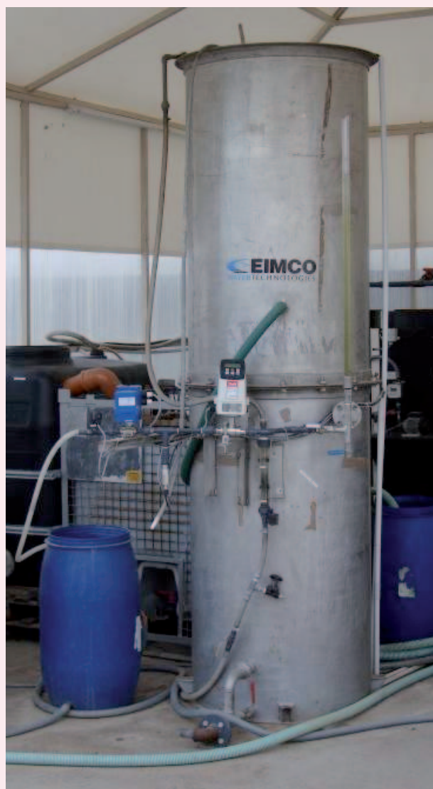
Figure 2: Photo of the pilot MBR installation
