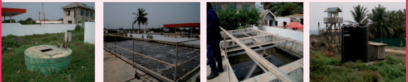
Figure 1. A WWTP (activated sludge) being operated in Accra, Ghana [From left to right; Stabilization tank, Aerated reactor, Settling tank and treated water tank, reused for lawns irrigation. Real flow rates: about 25 m 3 /h].
