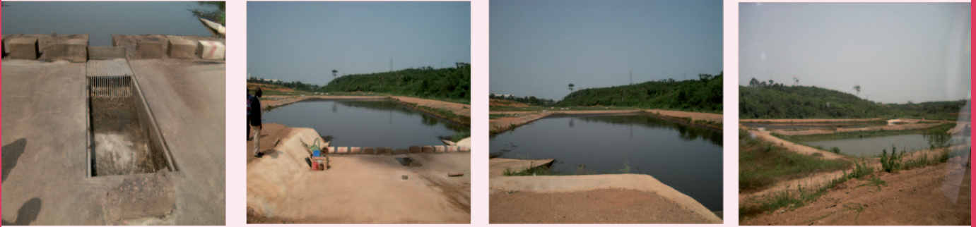
Figure 3. A faecal sludge treatment plant (pond system) in Sekondi-Takorady, Ghana. From left to right; Faecal sludge discharge area (from trucks); Series of ponds. Treats about 100 m 3 /d of faecal sludge.
