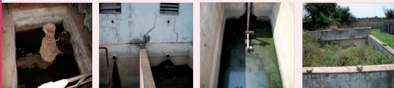
Figure 6. A WWTP in disrepair in Accra, Ghana. From left to right; pump, aerated reactors, settling tank, weedy drying bed.
