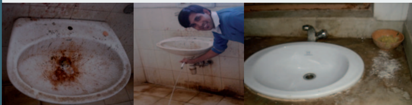
Figure 3: Pictures showing the conditions of wash basins at the toilets
