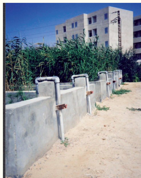
Figure 3: Effluent sampling points at the 6 1st stage HSSF beds
