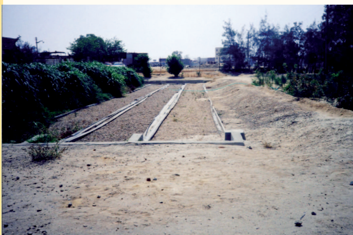
Figure 2: 1st stage HSSF beds, CW system in Ismailia, Egypt
