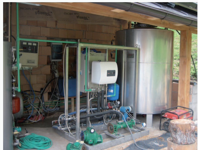
Figure 9: The biogas plant (Picture: G. Langergraber).
