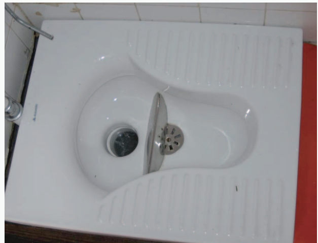
Figure 7: Squatting type separation toilet for daily visitors (Picture: G. Langergraber).
