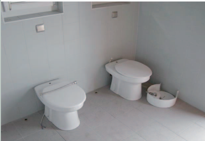
Figure 4: UDDTs (left, without separation walls) and urinals (right) during installation (Picture: Amor, 2006).
