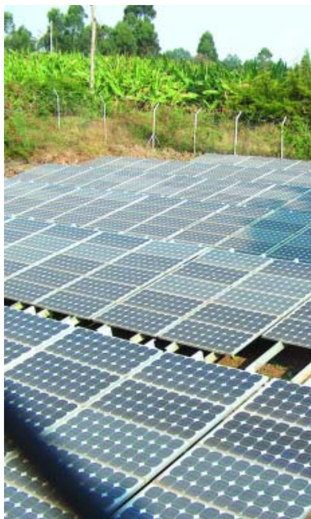
Solar pumping station for water supply system (Kisoro/Uganda)
